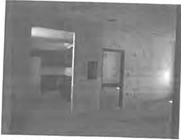
An interior view of a Bergen Court apartment during the rehabilitation process.
